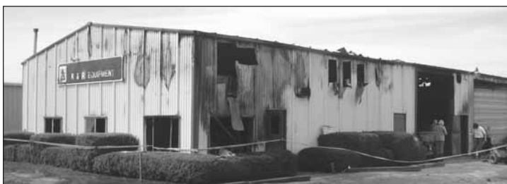
R&R Equipment in Indianola, Iowa suffered extensive damage from a fire in April. The dealership plans to rebuild and open this fall.
